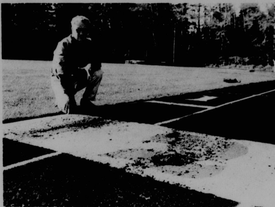
Track Coach James Hunt examines deteriorating track. — Photo by Randy Thieben
