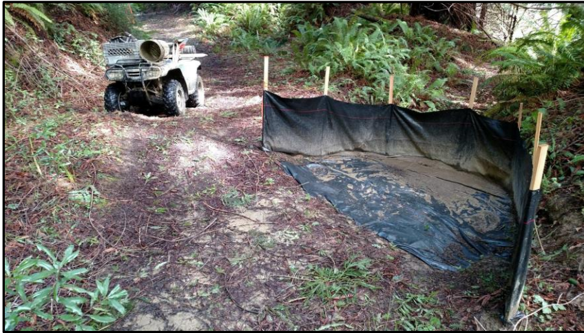
Figure 4. Silt fence on an inactive road segment with a slope class of 6-11 percent.
