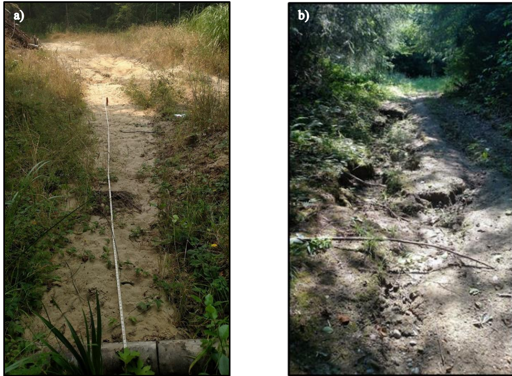
Figure 2. Measuring plume deposition below a waterbar (a), and rill/gully erosion on an inactive road segment (b).
