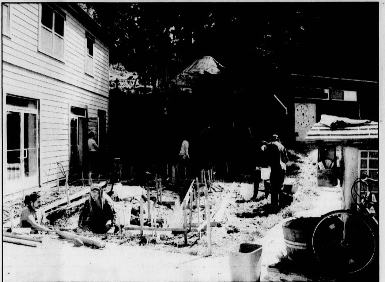
The Campus Center for Appropriate Technology has a “Volunteer Day” every Friday, where students and members of the community are welcomed to come and participate in many different kinds of projects. Pictured is the beginning construction of a greenhouse being built by students and volunteers. | Alyssa Alvarez
