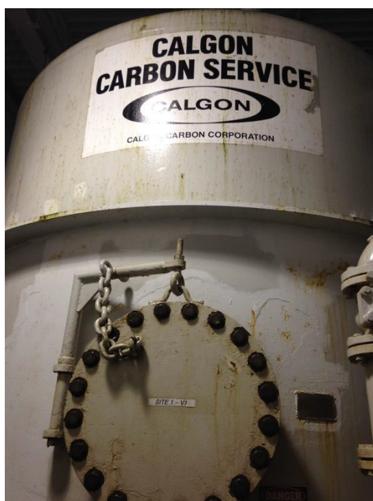
Figure 13 Carbon filter, managed by Glenn Springs Holdings (Revord, 2017)
