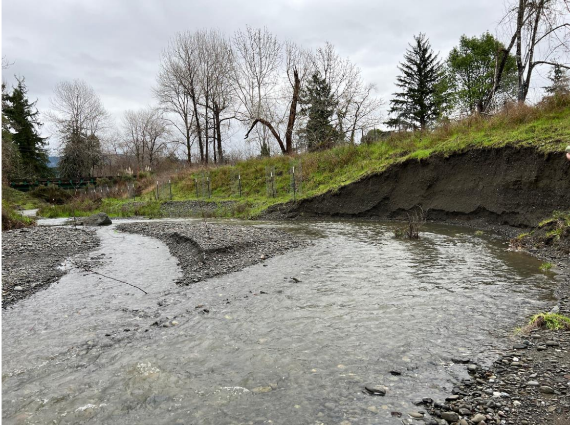
Figure 3: February 2024 post-erosion. Facing upstream Powers Creek with destabilized bank erosion on the right (Daniel Price).
