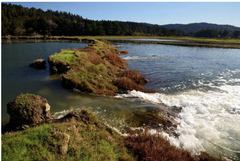
Dike overtopped during a King Tide inundating lands on South Bay 4
