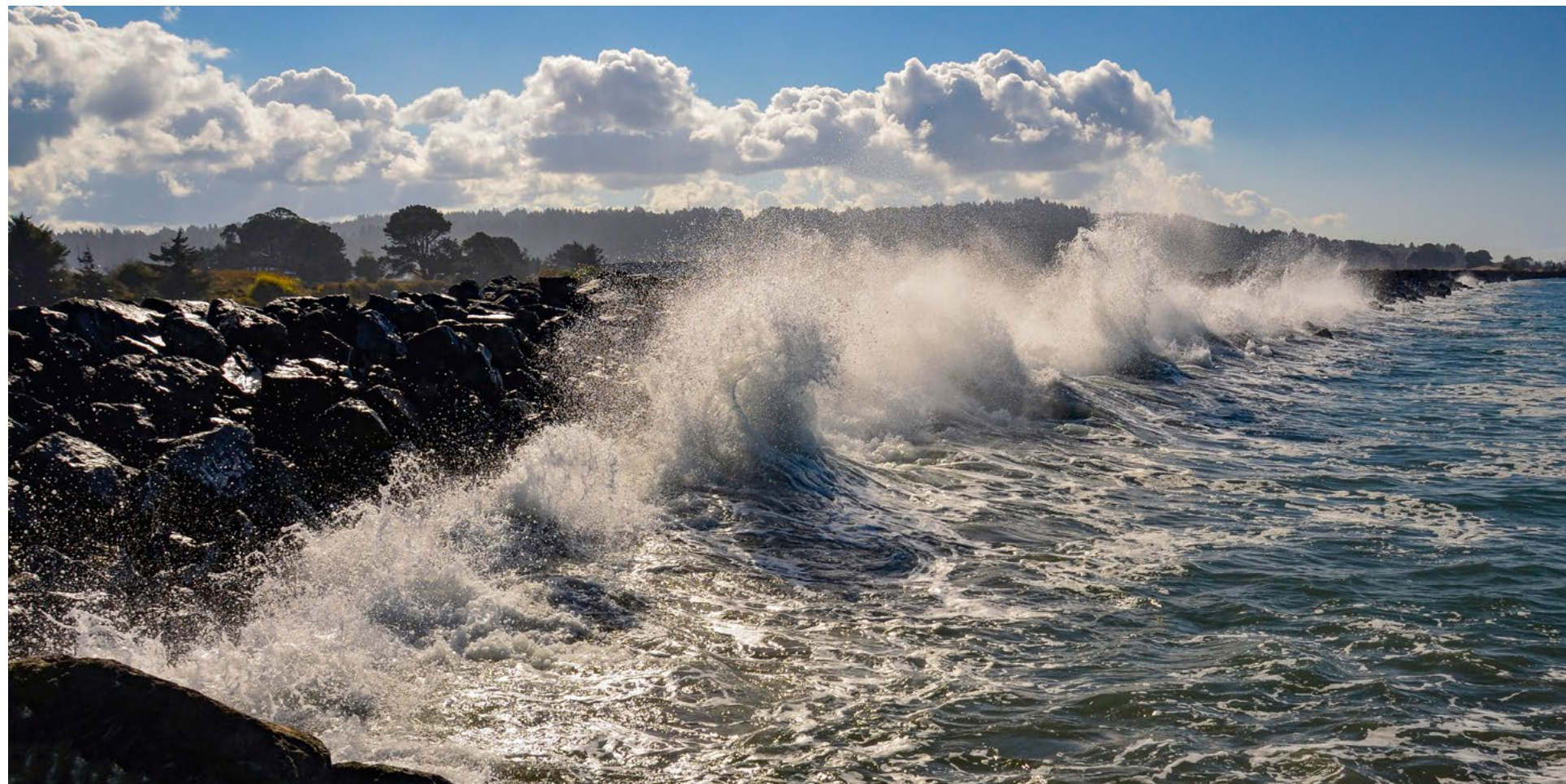
Sea wall receiving the full brunt of the waves funnelled through the north and south jetties on a not so calm day.
