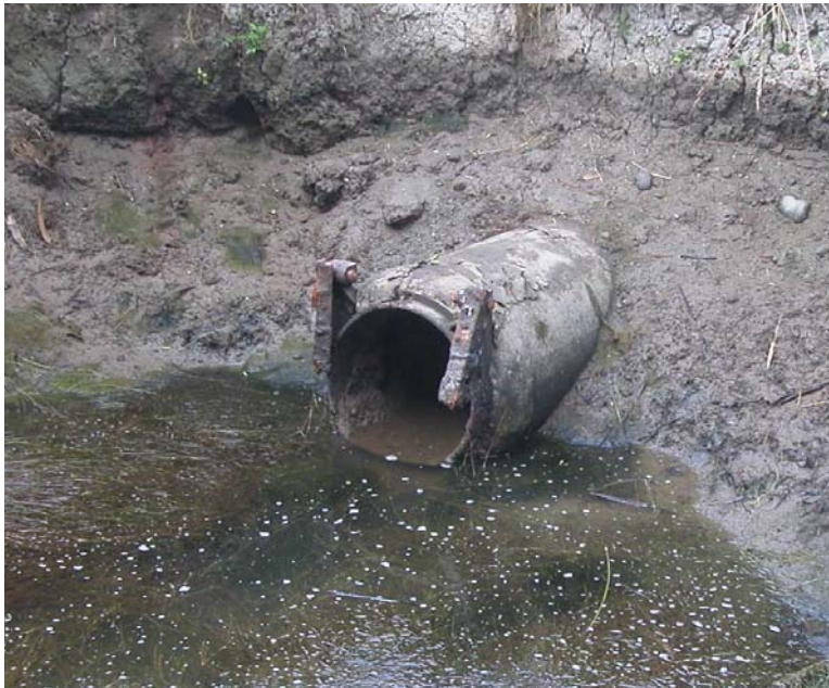
Figure 1. Example of a concrete pipe culvert with failed (missing) tidegate.
