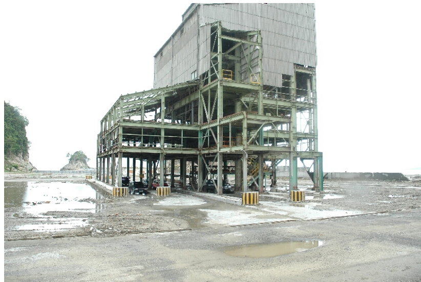
The curtain walls of the building were damaged, but the superstructure is intact. (SN 5/2005)
