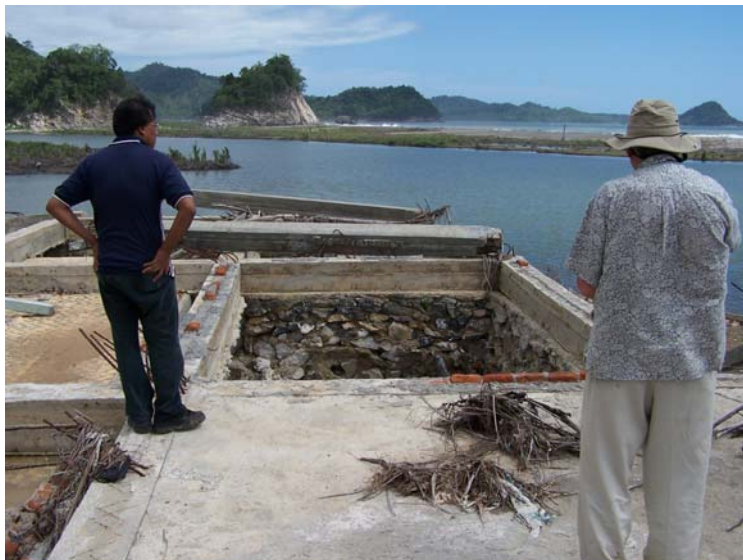
The buildings have been swept away but the foundation is intact and has little damage. (SN 5/2005)
