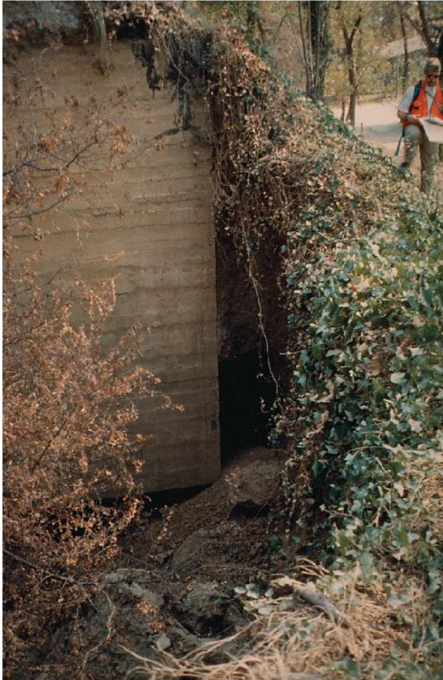
Right lateral displacement of over 2 meters displaced the soil around the bunker. The bunker twisted, but did not crack. (WDP 2000)
