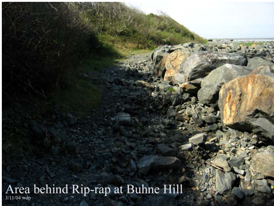
Swash has eroded local areas in rock along pathway. Buhne Point is in distance. (WDP 3/11/04).
