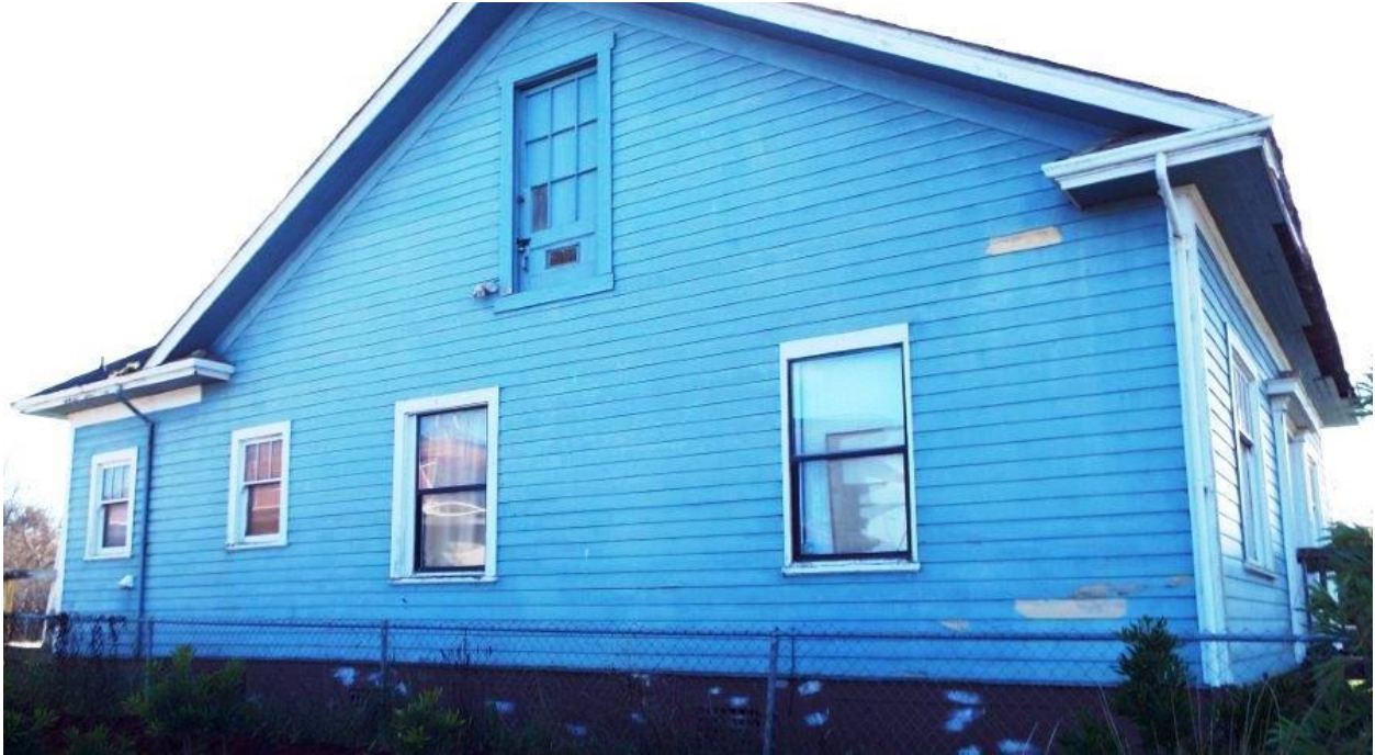
North elevation showing window changes and relocated door. Photo Jamie Roscoe Feb. 2015.
